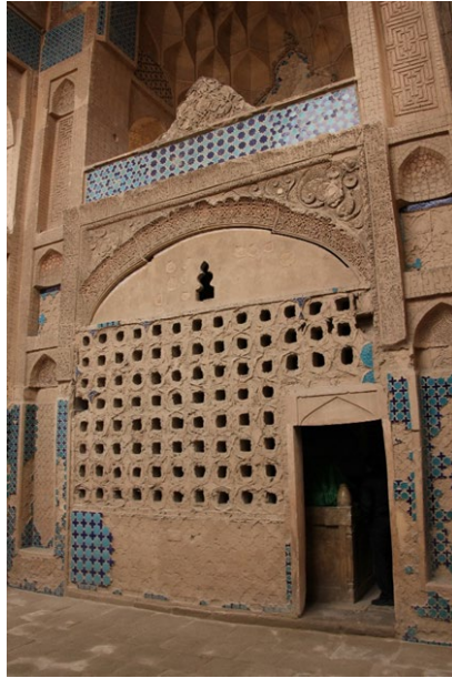
Img. 8: Grill separating the burial chamber of the Shaykh and the interior space of the iwan . The grill retains mortar for the adhesion of tile revetments. (Grbanovic 2018)
