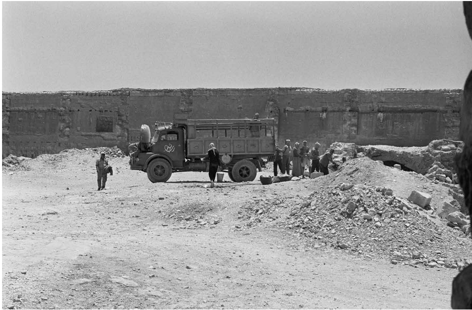
Figure 1.10. Workmen loading debris onto a dump truck, 1966 (Box 27, File #6, Negative Files 1964–1966, Sheet entitled “1966Z”).
