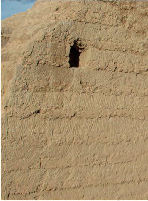
Fig. 42. The small northern niche high up on the east wall of Room 2.
